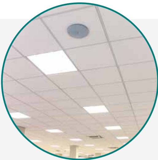
Application: Office light
